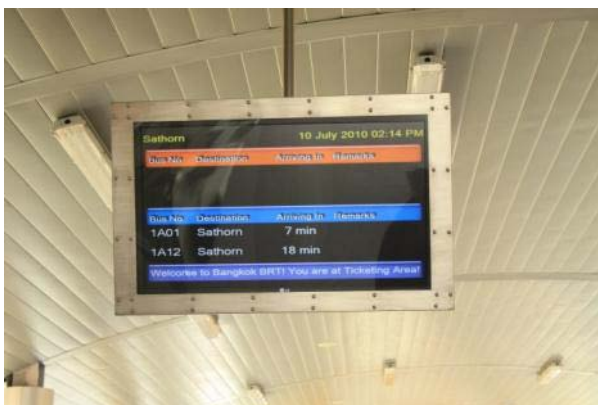
Figure 6: Information system at the BRT Sathorn station
