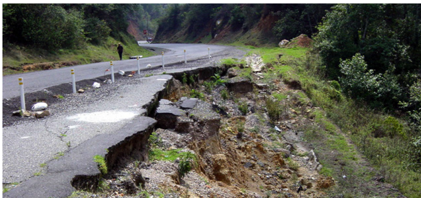
Figure 10 Flood damaged road in Guatemala.
